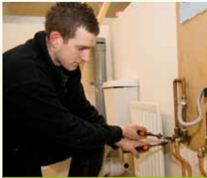
Plumbing Apprentice Brad Thomas competing for the title of Apprentice Plumber of the Year.
